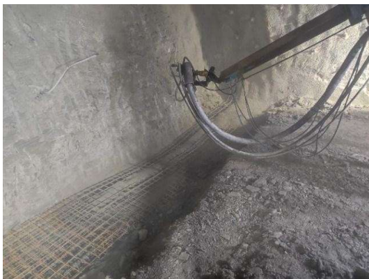
Figure 6. Installation of shotcrete on pre-reinforced II reinforcement zone/temporary invert (photo. N. Halilbegović, 2024)
