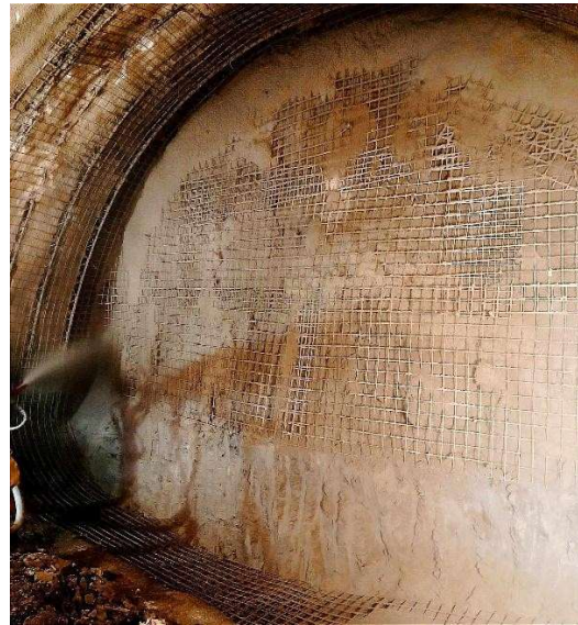
Figure 9. Installation of shotcrete on the pre-reinforced face of the excavation/top heading (photo by N. Halilbegović, 2024)
