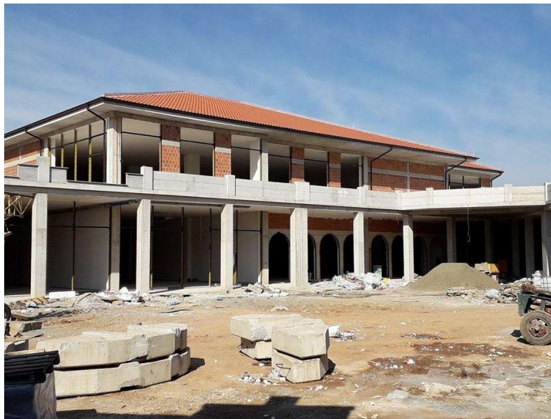
Figure 5: Presentation of the concept and context in the first phase of construction
