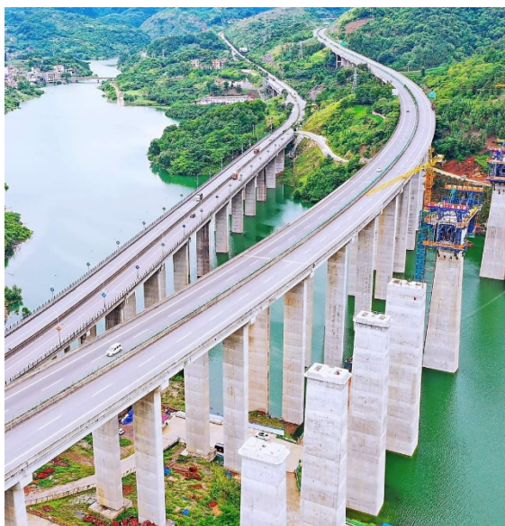
Figure 13. The construction site of the Nahuai River Bridge on the Panzhou-Xingyi High-speed Railway [16]
