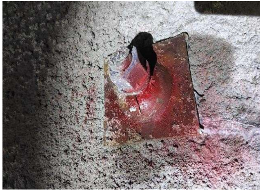
Figure 1. Condition of IBO anchor strain plate/crown (photo by N. Halilbegović, 2024.)
