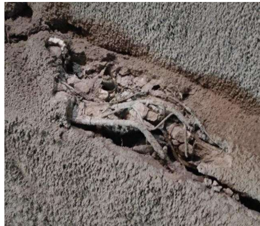
Figure 3. Condition of steel arch - grillage/crown (photo by N. Halilbegović, 2024.)
