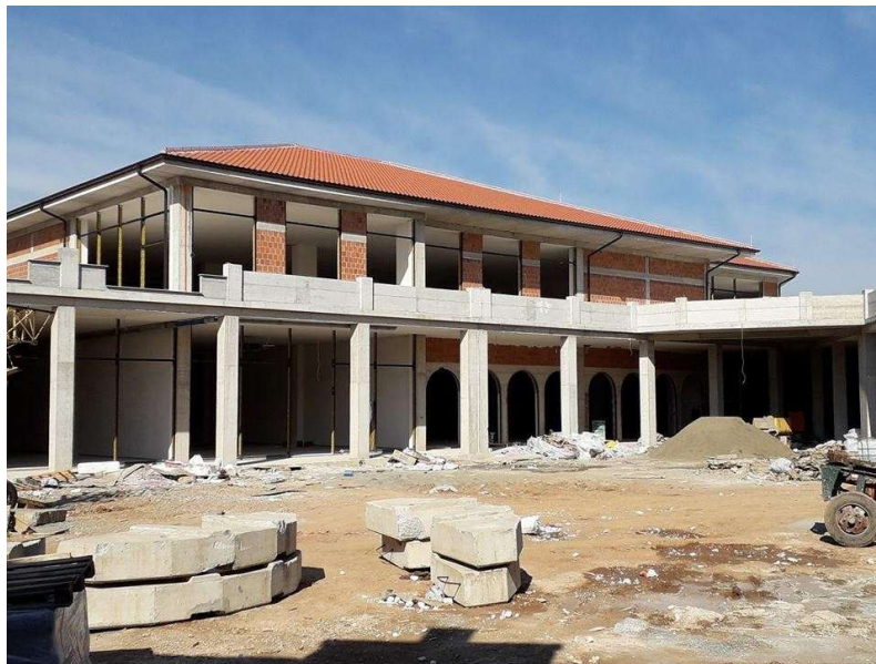
Figure 5: Presentation of the concept and context in the first phase of construction
